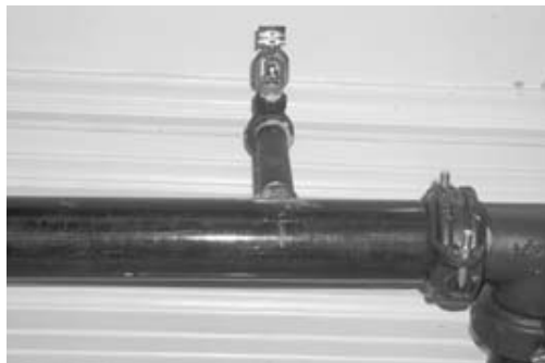
One of the 38 new sprinklers in the house.
